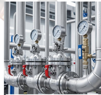
Stainless Steel – Valves and Gauges
